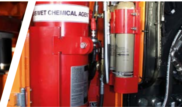
Automatic fire suppression system
